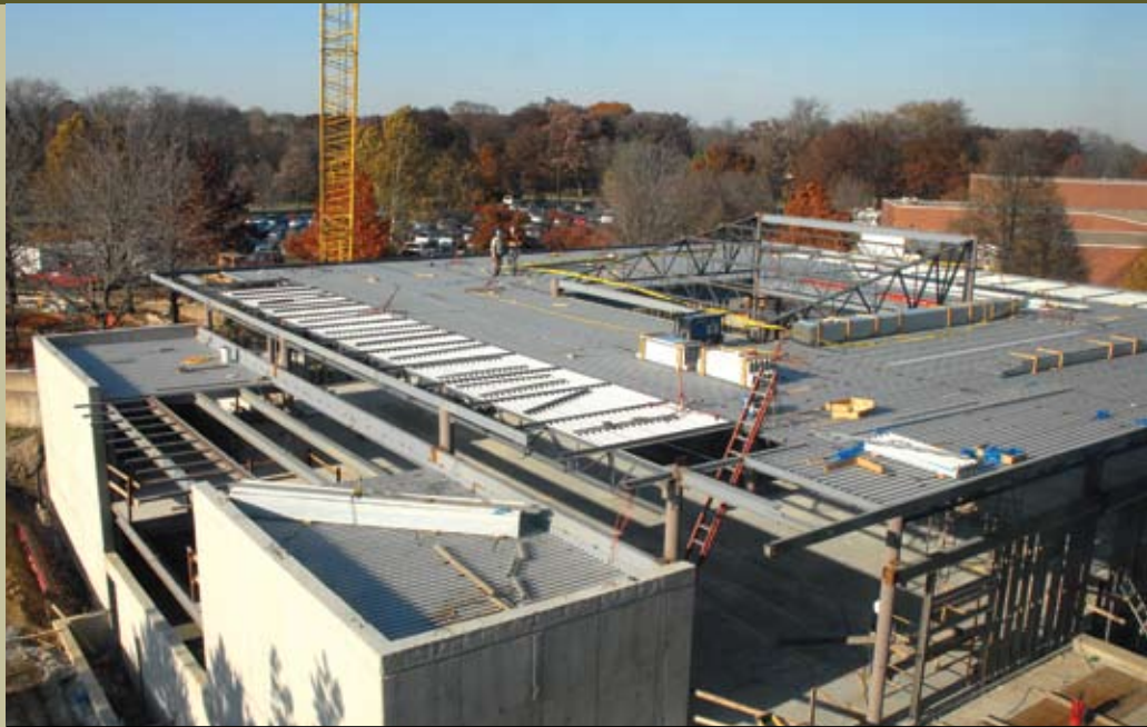
Construction crews took advantage of dry days in early November to make progress on the roof and walls of the pavilion. Photo by Heather Sauer.
